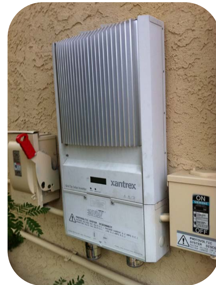
Inverter with DC and AC disconnect and wiring to building panel.
