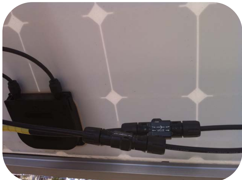
MC connectors between PV modules.
