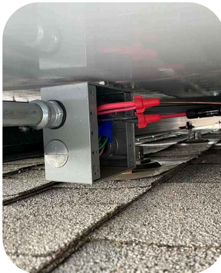
Transition from PV wire to wire in conduit to inverter.
