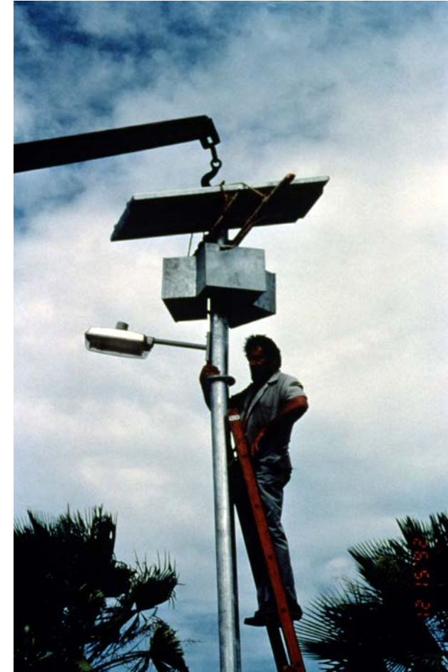
Worker installing a photovoltaic-powered street light in Brazil. Image by Roger Taylor / NREL 01860
