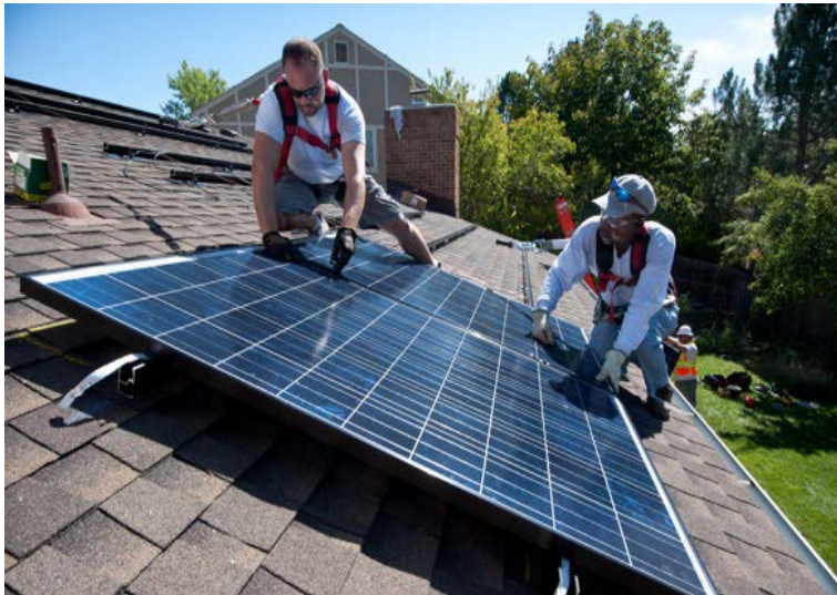
Photo by Dennis Schroeder, NREL 22168
