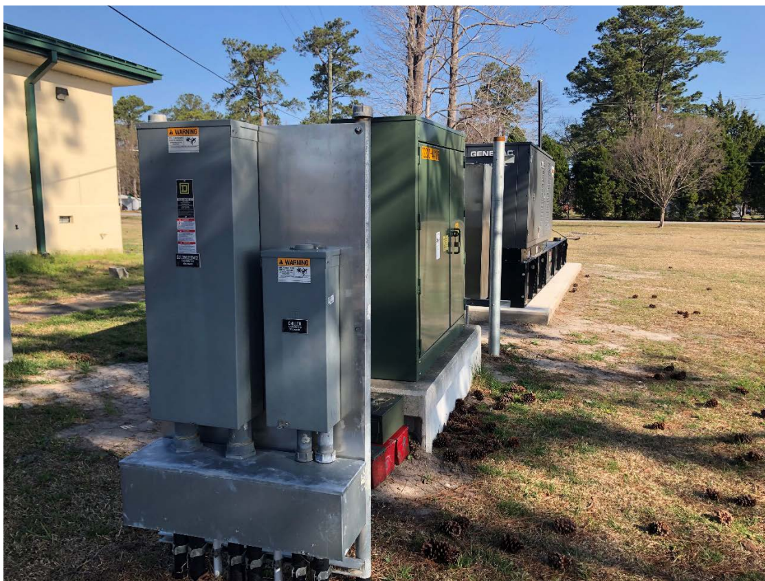
Figure 31. Transformer, panels, and generator behind AS-302
