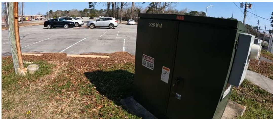
Figure 44. Building 895 parking lot and transformer
