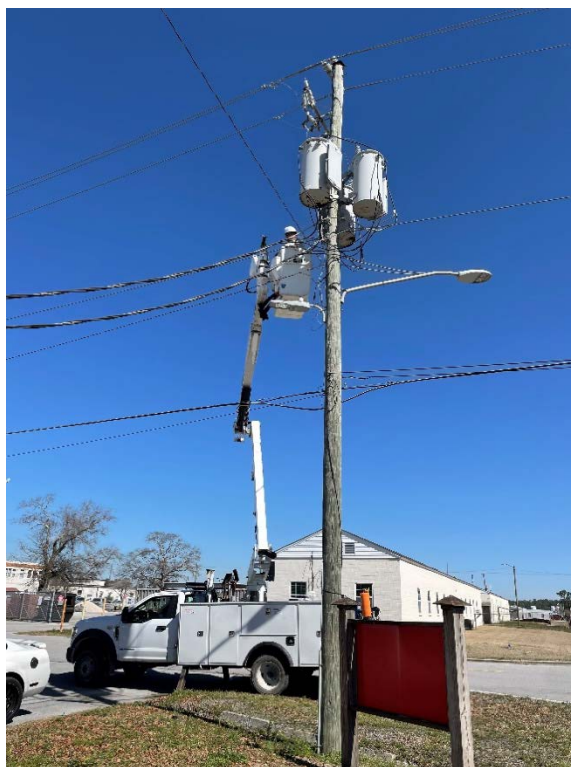
Figure 13. Sam Seaman checking power readings on Building 1308 utility pole
