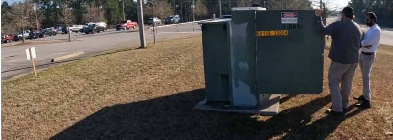
Figure 38. Ranjit Desai and Dale Swink by an existing transformer in Building B-329 parking lot
