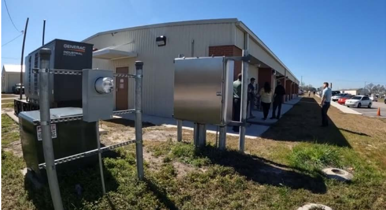
Figure 9. Transformer, generator, meter, and panel at the north corner of 1110 Ash Street
