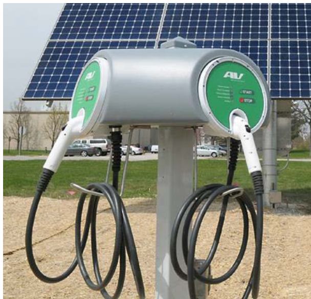
Figure 2. Dual-port pedestal EVSE unit
