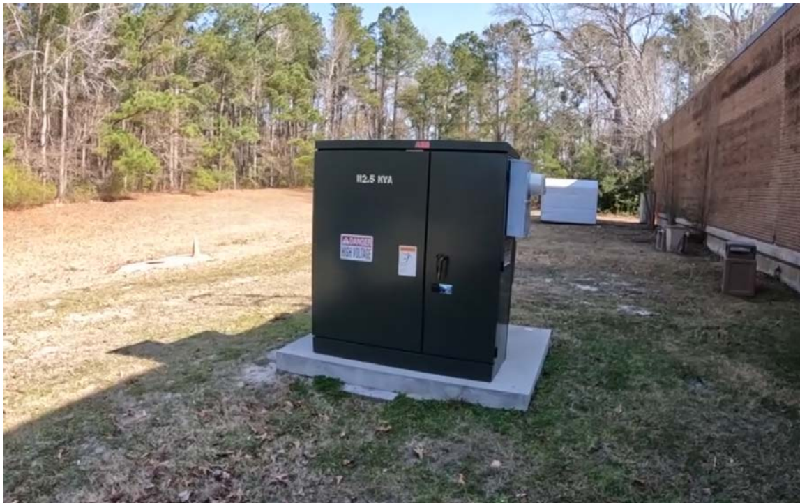
Figure 47. 112.5-kVA transformer behind Building 88
