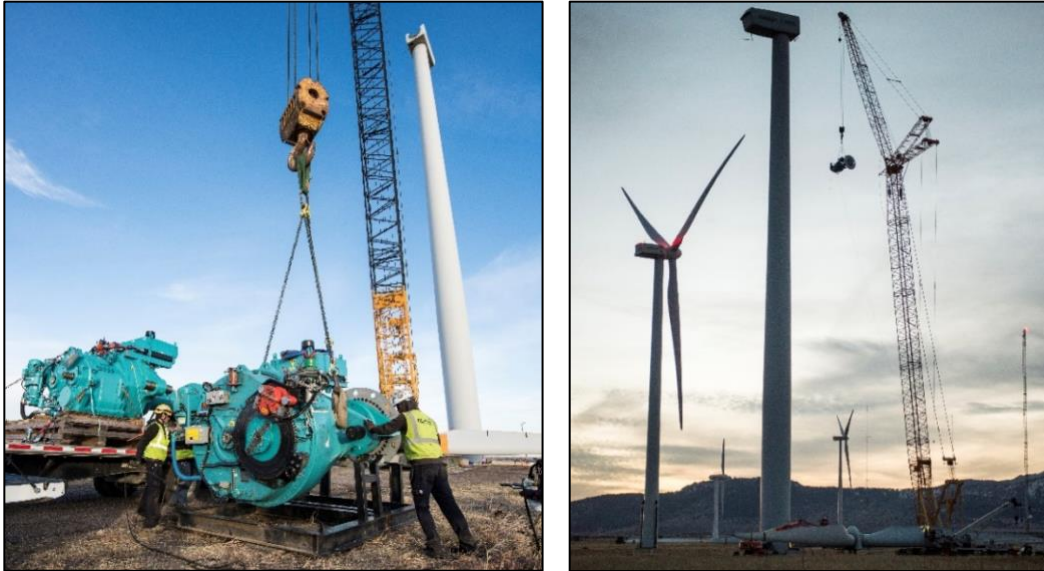
Figure 2. Gearbox swap (left) and installation in turbine (right). Photos by Dennis Schroeder, NREL 49409 and 49413
