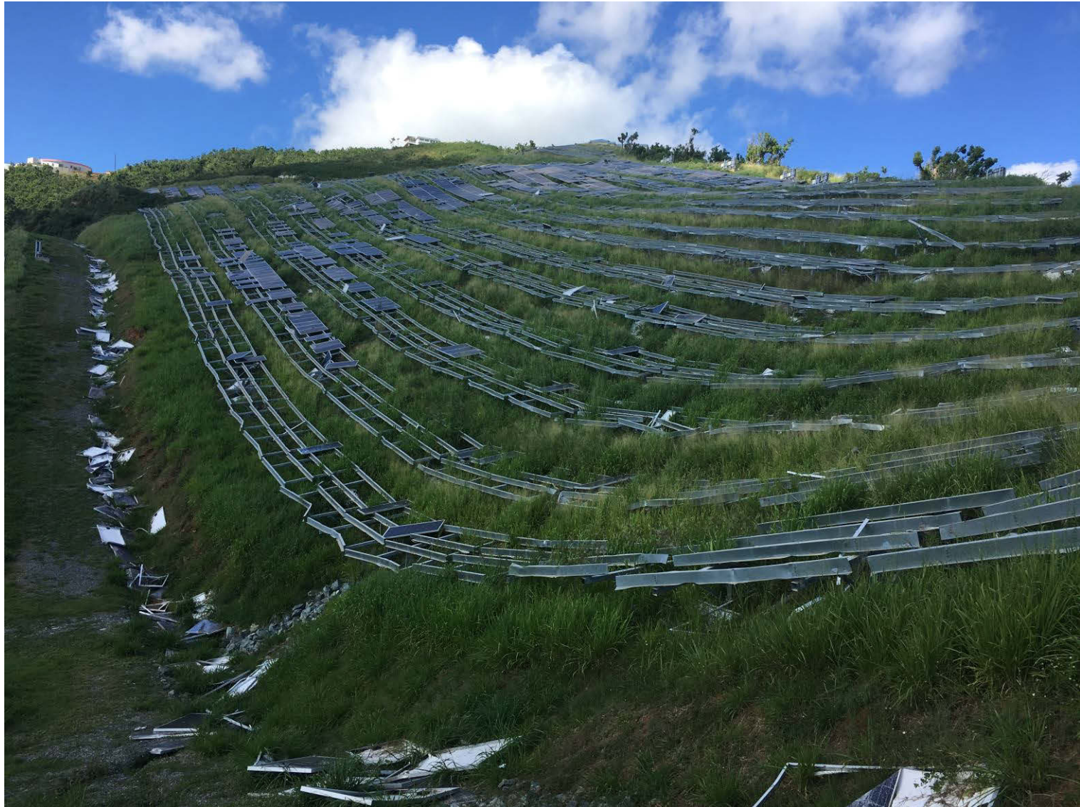
Same plant after Hurricane Irma, December, 2017
