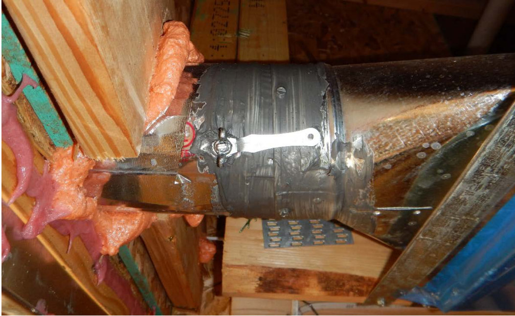
Figure 10. Register for the builder’s standard system, showing a balancing damper and mastic
