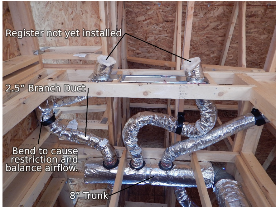
Figure 8. Small-diameter trunk-and-branch plenum on the third floor of Home A1
