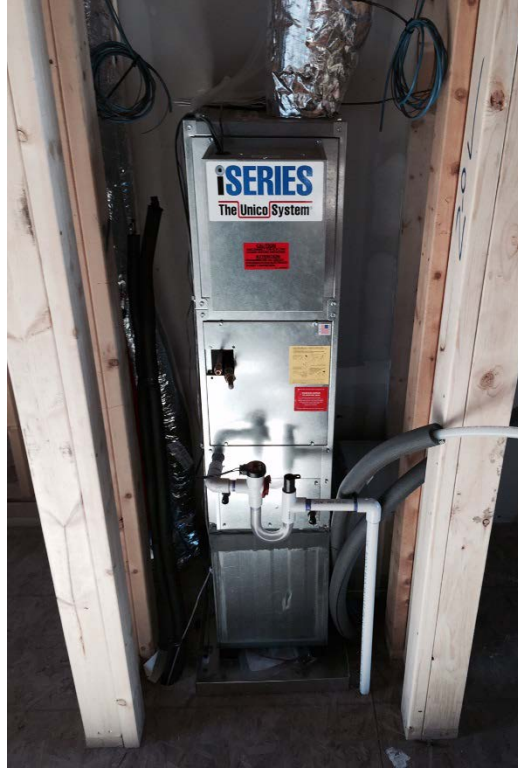
Figure 9. Small-diameter upflow air handling unit on the second floor of Home A2
