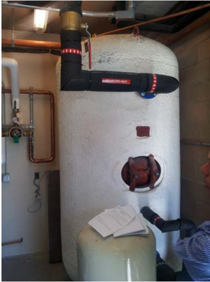
Solar storage tank, Site 1
