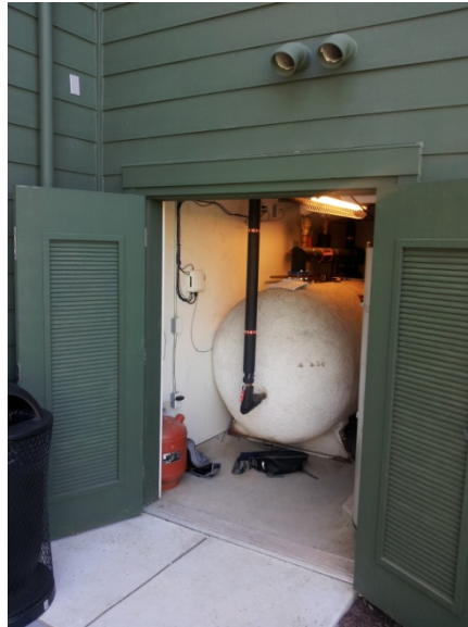
Solar storage tank, Site 2
