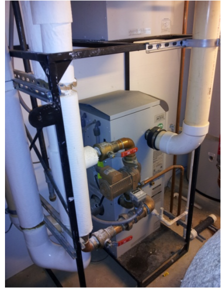
Condensing boilers heat water in insulated tanks
