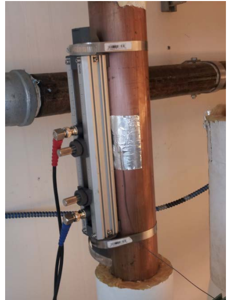
Ultrasonic flow meter and thermocouple installed on pipe for noninvasive monitoring
