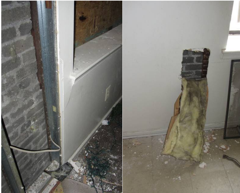
Figure 3. (L) View of wall assembly construction; (R) spot checks of the batt insulation showed poor installation and air movement within the wall cavity
