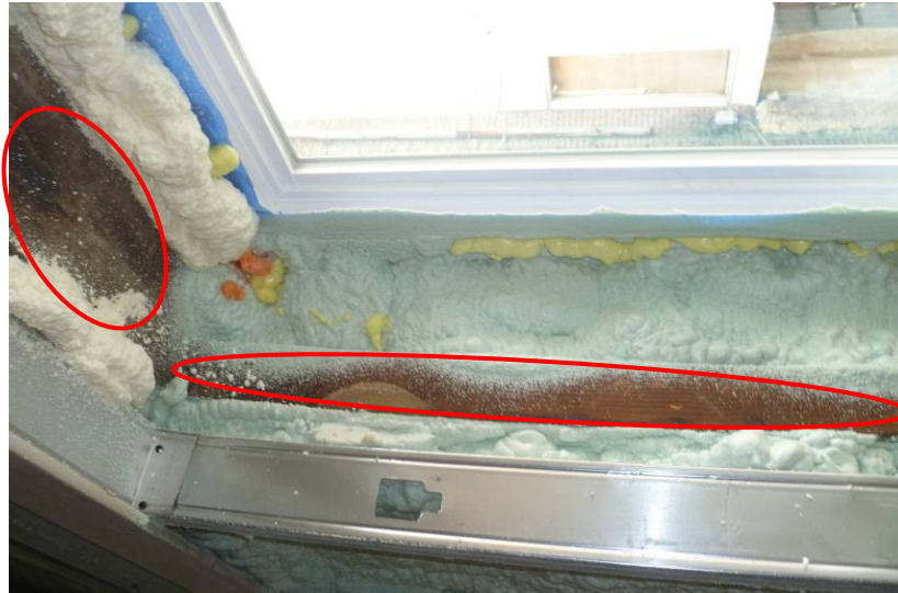
Figure 28. Missing ccSPF insulation around window rough opening
