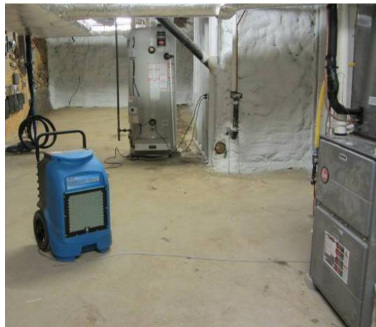
Figure 30. Stand-alone dehumidifier installed in a basement
