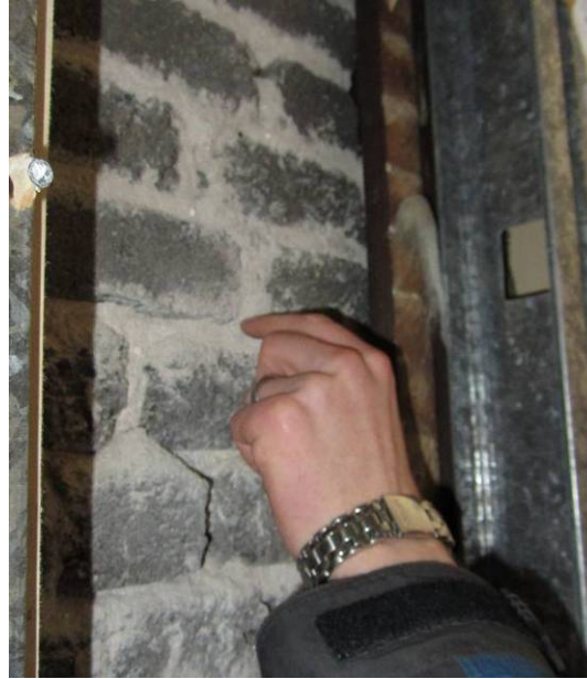
Figure 5. Brick mortar crumbling just from the touch of a finger
