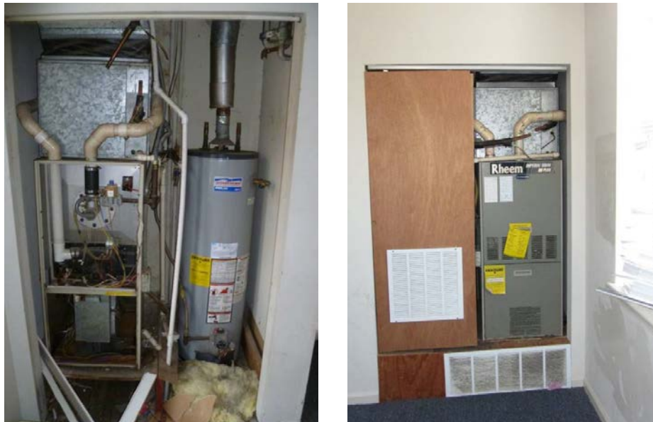
Figure 14. Atmospheric water heater located in furnace air handler closet with poorly sealed central return
