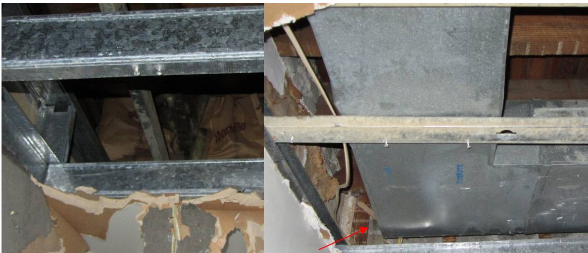
Figure 4. (L) Poor installation of batt insulation at the rim/band joists; (R) missing rim/band insulation due to ductwork obstruction
