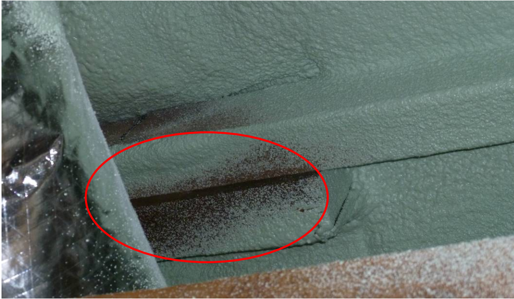
Figure 26. ccSPF should be applied to the whole length of these “sister” trusses to seal gap
