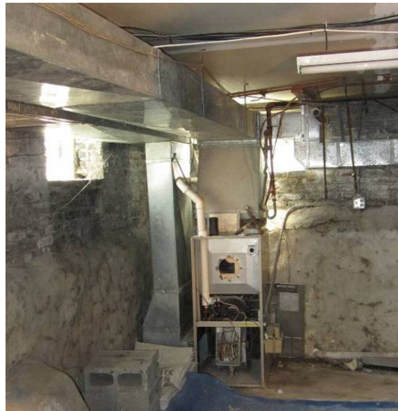
Figure 12. Uninsulated and leaky HVAC system for a first-floor apartment located in an unconditioned basement
