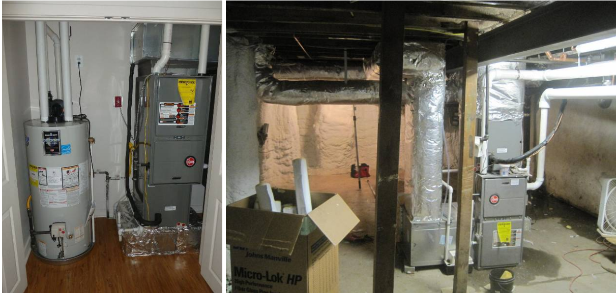
Figure 29. (L) The furnace and water heater do not draw combustion air from the interior and direct exhaust flue gases to the exterior, so the risk of CO spillage has been drastically reduced. (R) This HVAC system located in a basement has been brought within the thermal envelope of the building and ductwork has been air sealed and insulated.
