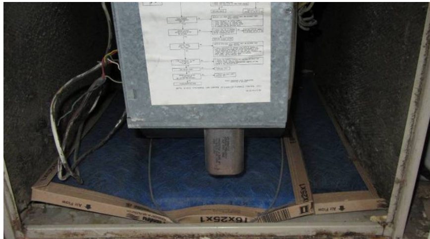
Figure 15. Improper air filters installed into existing furnaces
