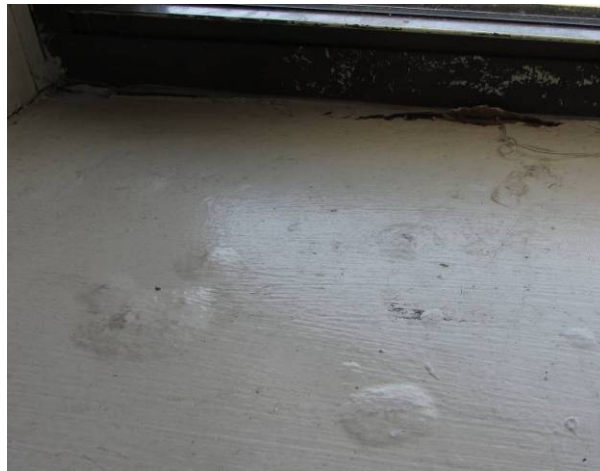
Figure 6. Bubbling of paint on window sill
