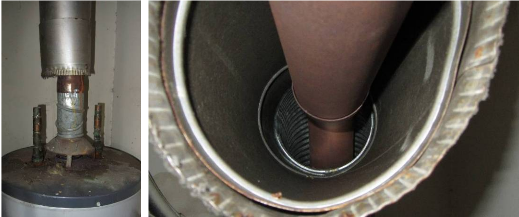
Figure 13. Make-up combustion air being provided for the water heater
