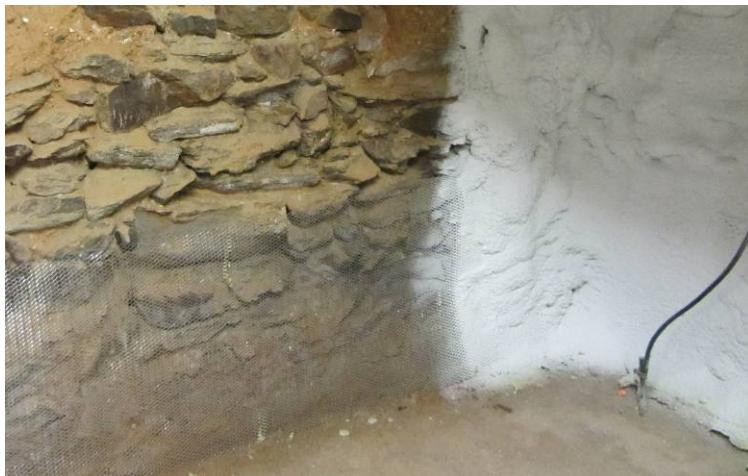
Figure 21. Wire mesh applied to bottom of stone foundation wall to help secure ccSPF in place
