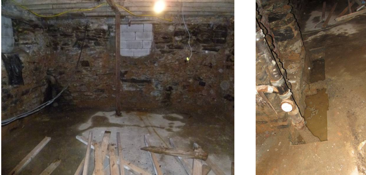
Figure 7. (L) The existing foundation has moisture issues with water intruding through the foundation walls and slab. (R) When additional footing supports were being dug, it was clear that the water table is quite high in this area.
