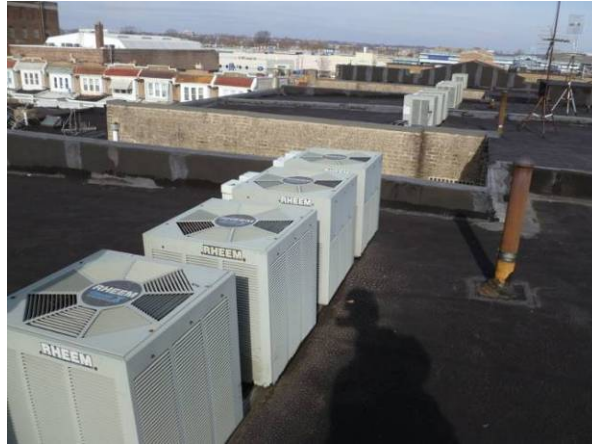
Figure 11. A/C condensing units on rooftop
