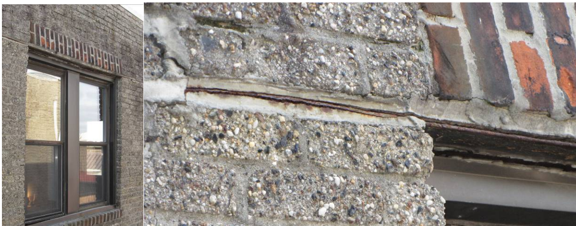
Figure 10. Deflection of steel angle window header
