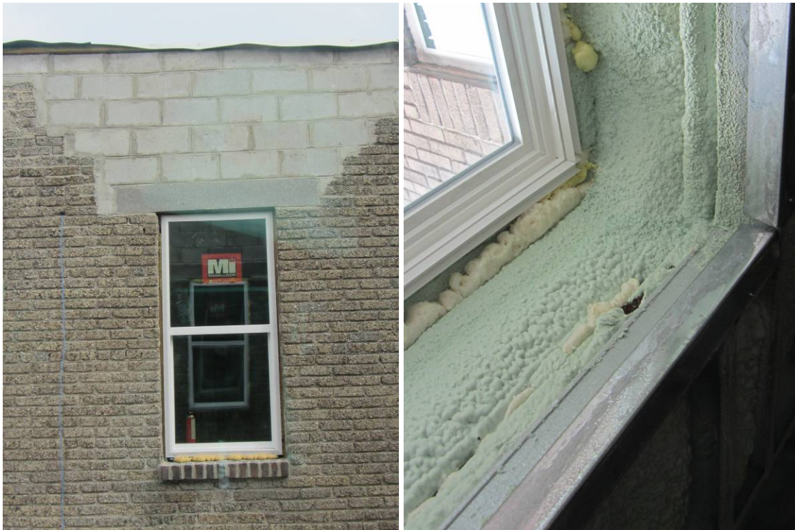
Figure 24. (L) Rebuilt window header; (R) ccSPF applied to rough opening to air seal and insulate
