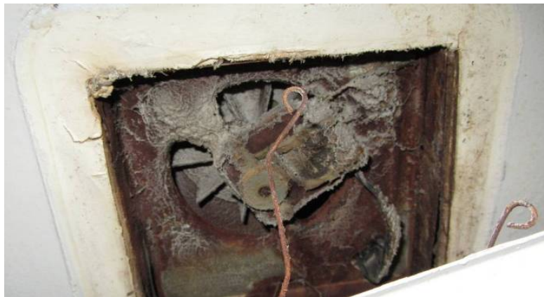
Figure 16. Condition of existing bathroom exhaust fan
