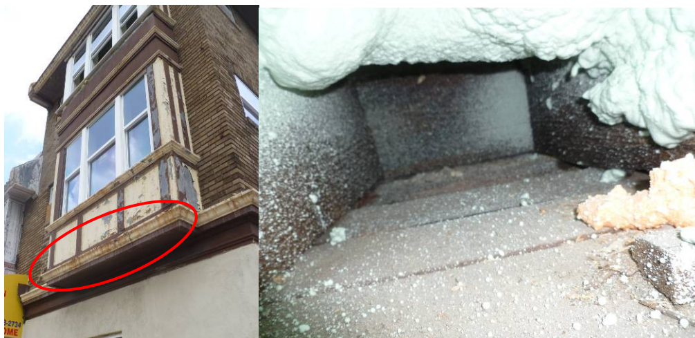
Figure 27. (L) Location of thermal/air bypass in exterior wall bump-out; (R) Looking from the interior ceiling out into the floor overhang of the window bay
