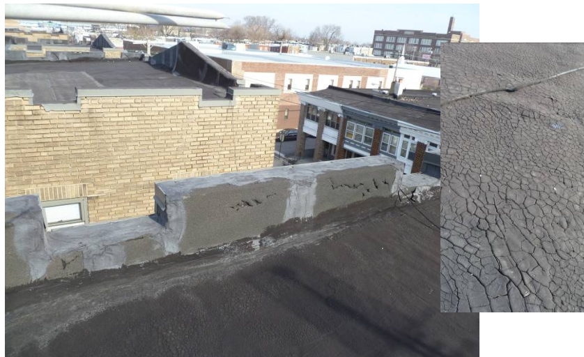
Figure 8. Deterioration of roof as evidenced by “alligatored” asphalt coating and degraded coating on parapet
