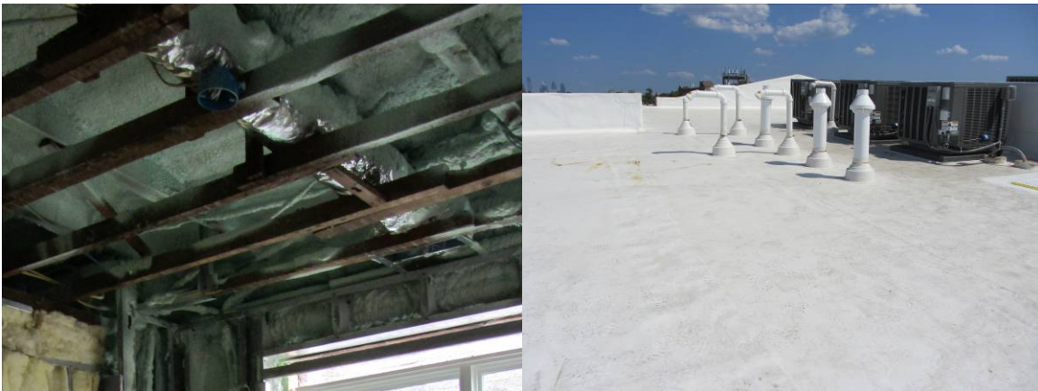
Figure 23. (L) 3 in. of ccSPF applied to underside of roof deck; (R) 3 in. of polyisocyanurate applied over the roof deck and covered with a white TPO membrane
