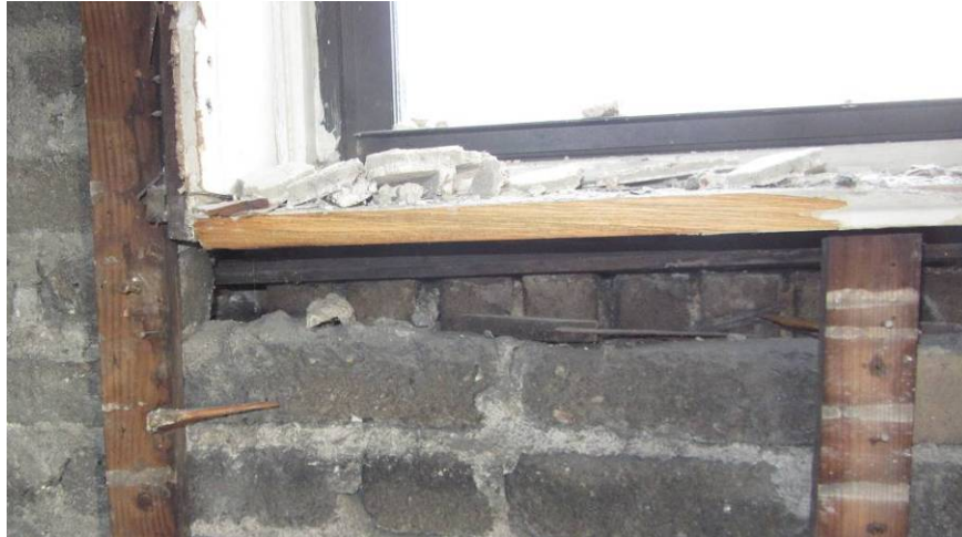
Figure 9. The inner course of brick was removed when installing the windows back in the 1990s renovation
