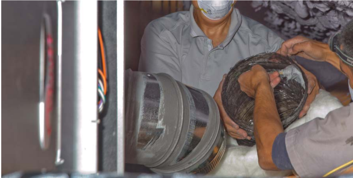
Figure 26. Mastic being applied to inside of flexduct jacket before being slipped over and secured to a branch takeoff elbow with compression bands
