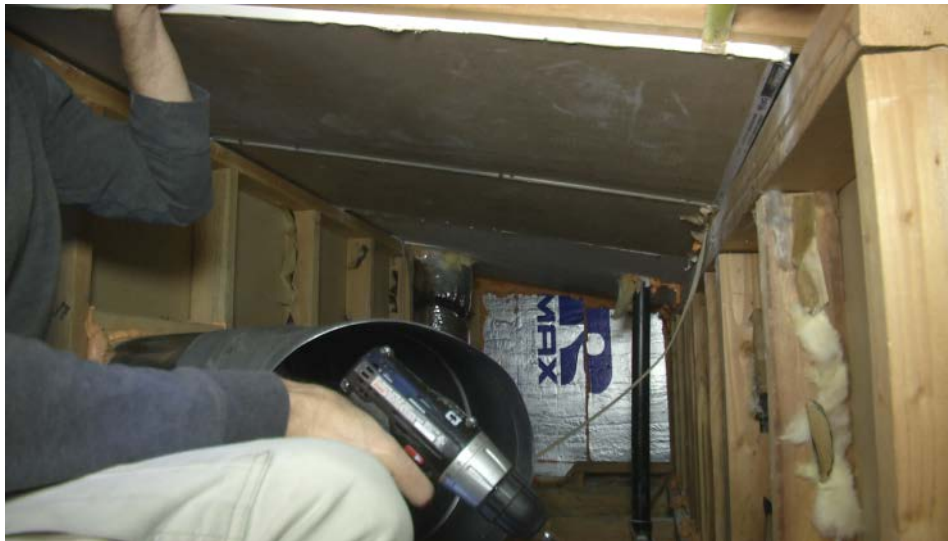
Figure 29. Pressure boundary being moved up to the bottom of the scissor trusses to allow ducts to remain within the building envelope
