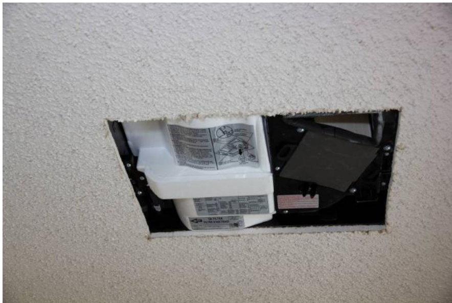
Figure 23. Spot ERVs installed in both homes to provide balanced whole-house ventilation
