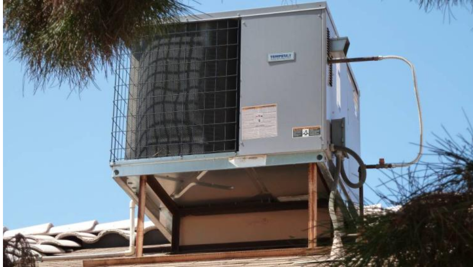
Figure 15. Rooftop packaged furnace/AC located at the Sierra Hills home (Image courtesy of Building Media, Inc.)
