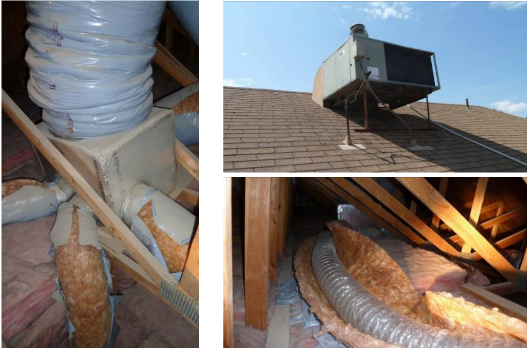
Figure 8. From left clockwise: supply plenum located in the vented attic, roof-mounted packaged furnace/AC, and insulation unwrapping from flex duct because the exterior vapor barrier had deteriorated
