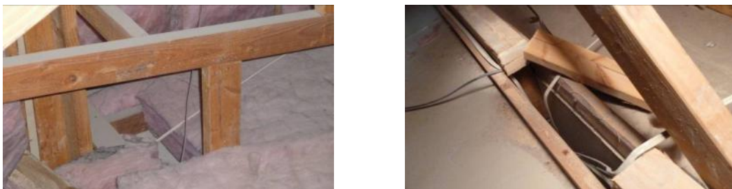
Figure 4. Top plate of interior walls cut out for electrical runs into partition walls
