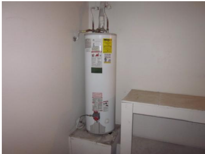
Figure 16. Atmospheric water heater located in the garage of the Sierra Hills home (Image courtesy of Building Media, Inc.)
