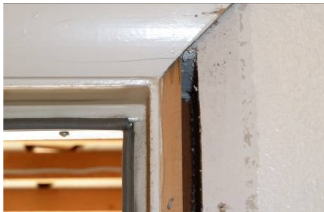
Figure 7. Lack of air sealing around exterior doors
