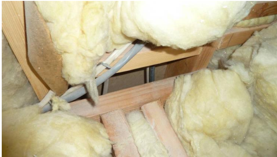
Figure 14. Interior wall cavities that are directly communicating with the attic
