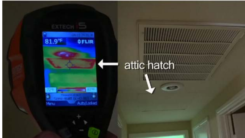
Figure 12. Leakage in ceiling plane (Image courtesy of Building Media, Inc.)
