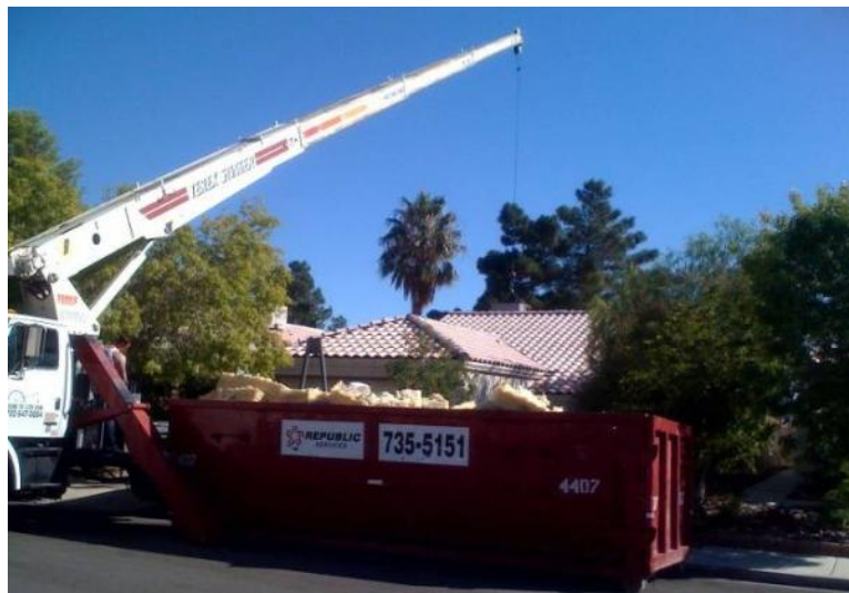
Figure 21. Existing package furnace/AC unit being craned off of the Sierra Hills home (Image courtesy of Building Media, Inc.)
