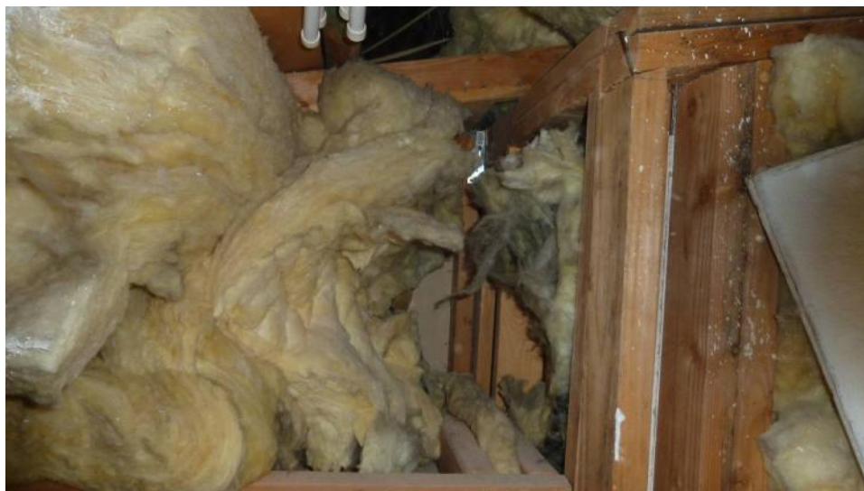
Figure 13. Poor insulating of partially vaulted ceiling kneewalls (Image courtesy of Building Media, Inc.)
