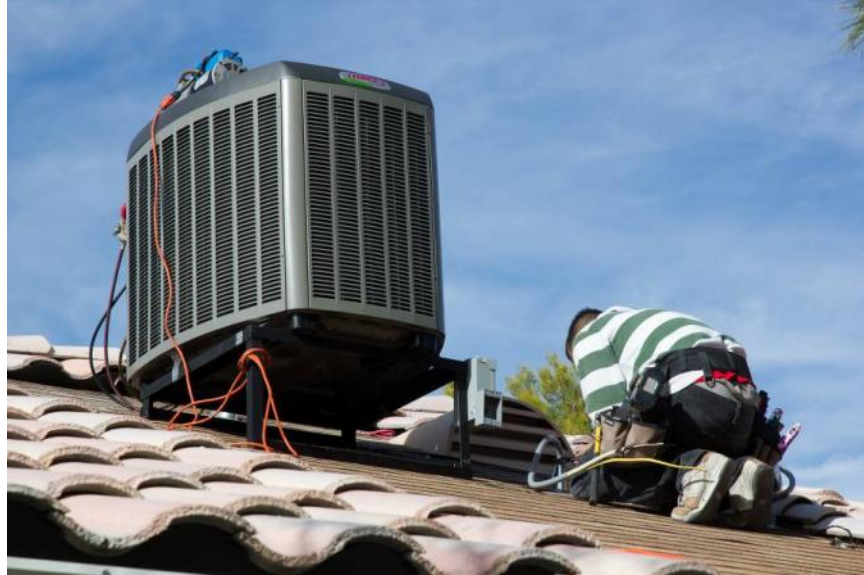
Figure 22. New outdoor heat pump unit being installed at the Sierra Hills home
