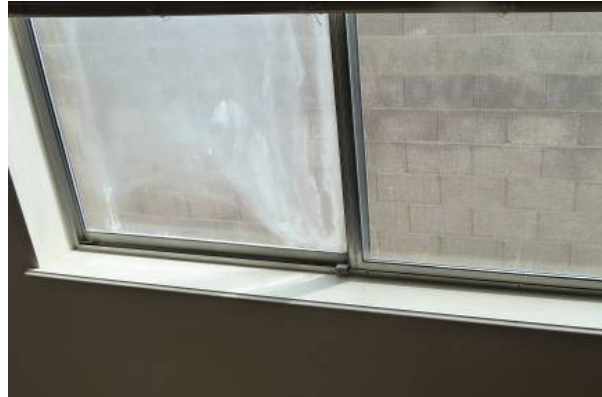
Figure 6. Haze between the window panes is evidence of a broken hermetic seal
