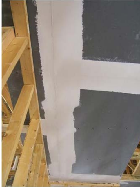
Figure 4. Drywall is also offset beyond the wall/chase to allow for marrying adjacent drywall
