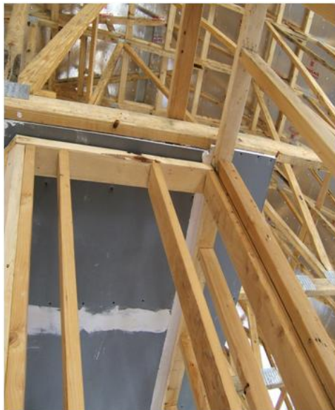
Figure 3. Drywall slipped through \frac{3}{4} -in. space between the top plate of the nonload-bearing interior wall
