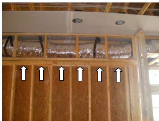
Figure 5. Arrows point to code-required fire blocking under chase, preventing insulation from being easily installed behind duct. Correction involves re-sequencing so insulation can be installed in this area prior to duct.
