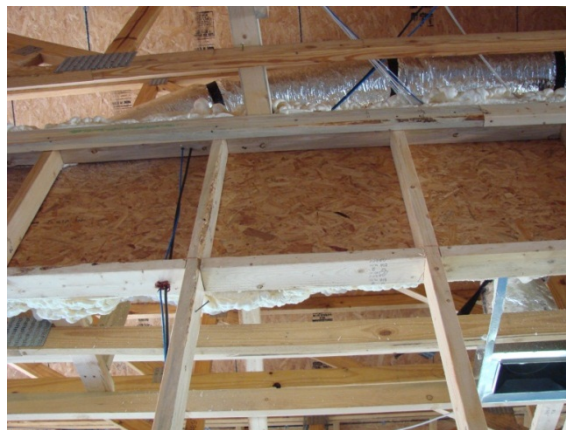
Figure 6. Backside of a foamed knee wall, showing blocker board used to serve as backing for the foam
