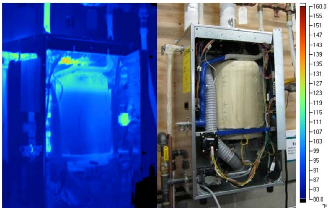
Figure 10. Infrared and visual images of TWH 2 in standby operation
