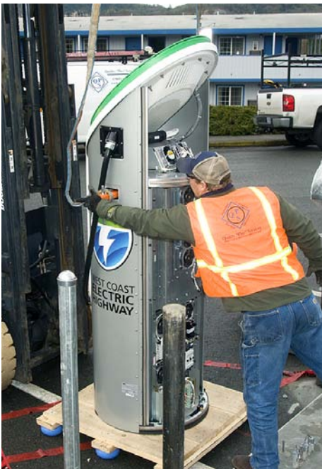
Workers install charging equipment in Grants Pass, Oregon. Photo from ODOT Photo and Video Services, NREL/PIX 20643
