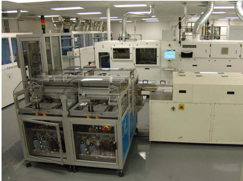
Figure 18: Integrated Ink-jet printer/dryer after installation at Innovalight; the printer is on the left and the dryer system is on the right side
