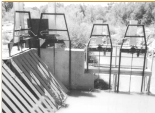
The Bureau of Reclamation uses PV to power motors that operate automatic gates for water flow control in irrigation canals. These systems improve the efficiency of water use and eliminate the need for Bureau personnel to manually operate the gates each day. NCPV researchers at Sandia are working with the Bureau to develop system diagnostics and communications systems.
