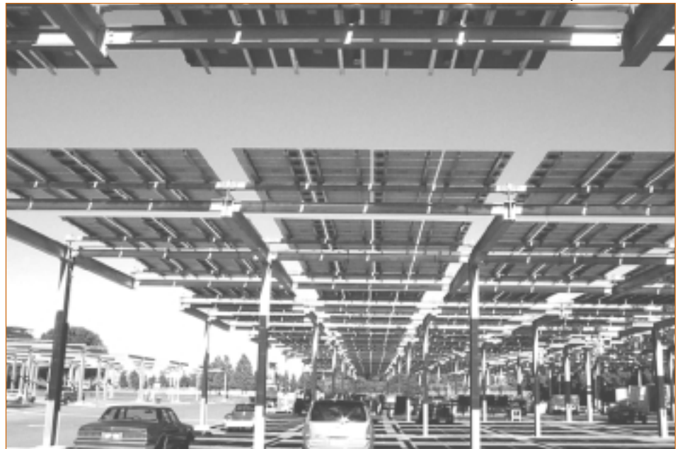
This solar electric system in Sacramento, California, generates enough electricity to meet the needs of about 180 homes. While providing electricity, it also shades part of the Cal Expo parking lot. The largest parking-lot solar system in the world, this project was a joint effort of the Sacramento Municipal Utility District and DOE through the TEAM-UP program.
